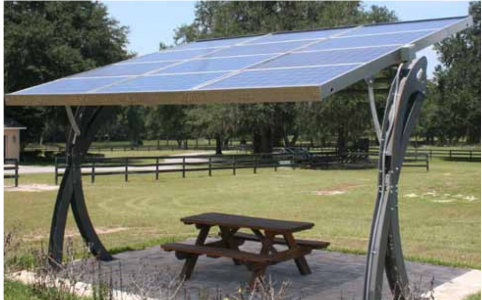
Courtesy Dan House Electric (2)
